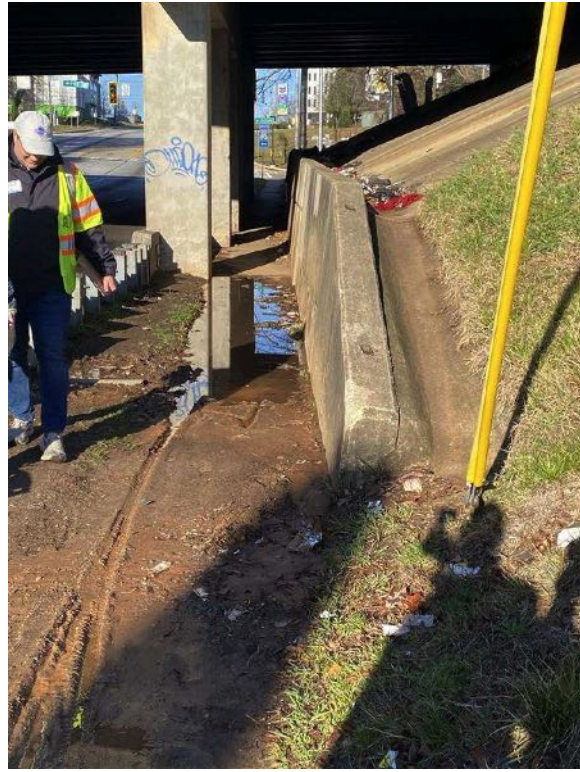
PHOTO 10: DRAINAGE ISSUES AFFECTING WALKING CONDITIONS UNDER THE CLEVELAND AVENUE AT I-85 BRIDGE
