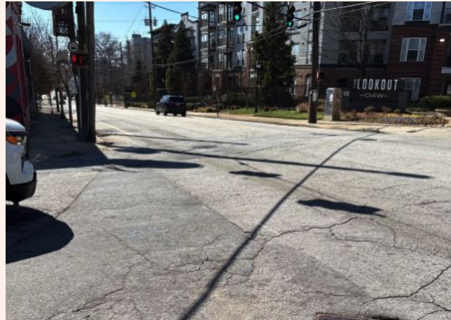
7 Intersection lacks crosswalks and adequate pedestrian infrastructure; drivers fail to stop for crossing pedestrians.
