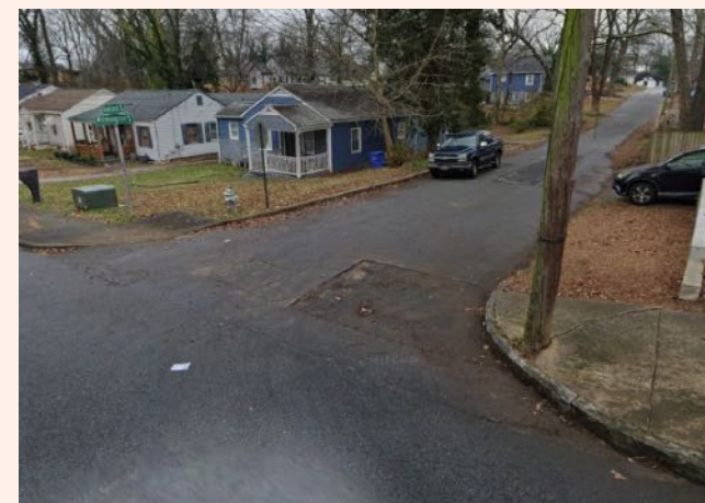
15 Missing sidewalk ramps on Oakland Dr SW.
