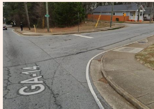
22 Existing sidewalk ramps not ADA compliant at Oakland Ln SW/Lee St SW.
