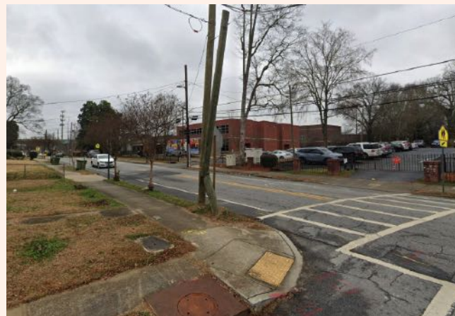
34 Broken utility poles throughout study area.
