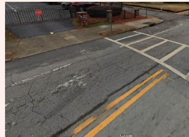
1 Faded striping, crosswalks, and pavement markings, including "SCHOOL" markings on Avon Ave SW.
