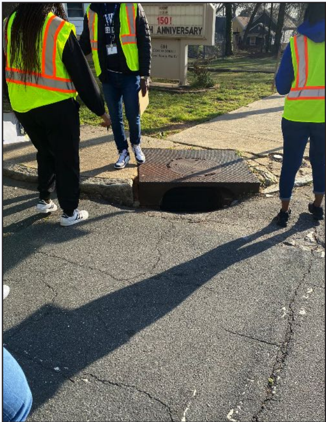
Stakeholders expressed concern uncovered drain inlets
