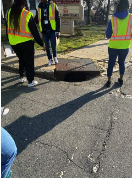
PHOTO 9: MISSING DRAIN INLET COVER AT THE INTERSECTION OF GLENN STREET AT COOPER STREET
