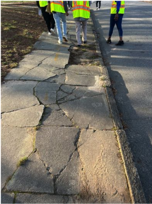
PHOTO 1: DAMAGED SIDEWALK ALONG WHITEHALL TERRACE, SOUTH OF THE SCHOOL
