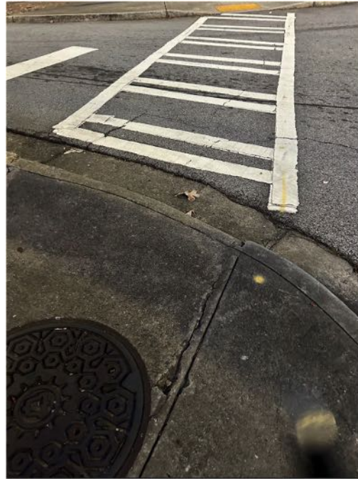
PHOTO 8: MISSING ADA CURB RAMP AT THE INTERSECTION OF FULTON STREET AT WHITEHALL TERRACE
