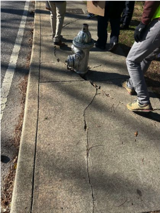
PHOTO 3: CRACKED SIDEWALK ALONG OLD HAPEVILLE ROAD
