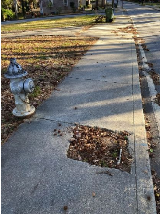
PHOTO 9: SIDEWALK MISSING AROUND WATER UTILITY COVER
