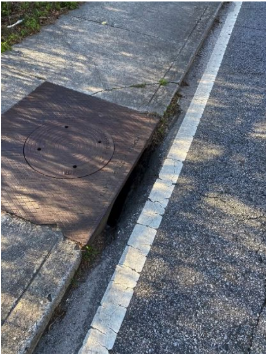
PHOTO 11: STORMWATER INLET MISSING GRATES
